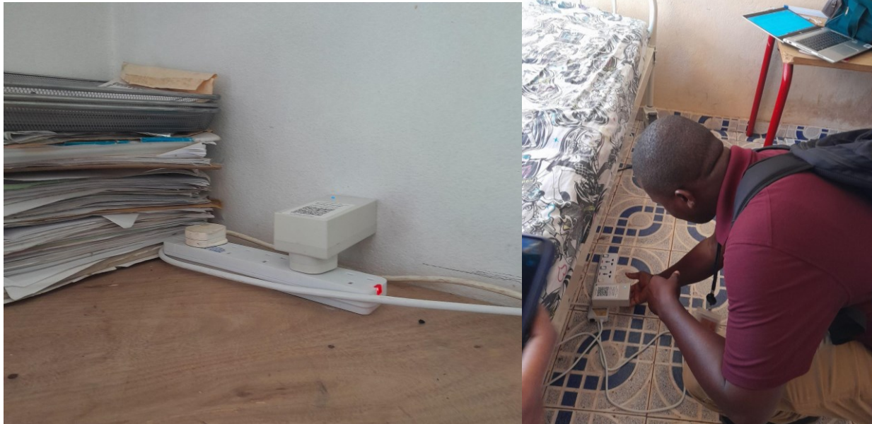
Figure 7: GridWatch sensors installed at Masanga Government Hospital. Each sensor is plugged into an nLine-provided powerstrip to ensure limited electric sockets are not taken by the sensor.
