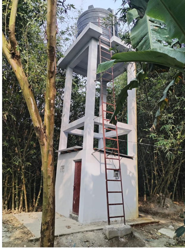
Figure 2: Water tower for pipeline network
