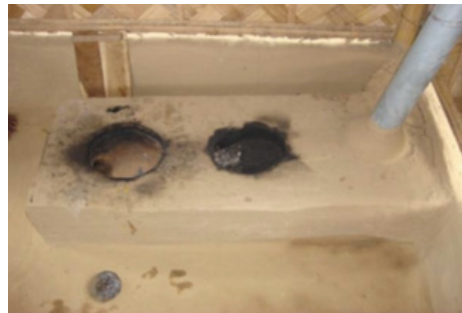
Left: Improved Chimney Stove
